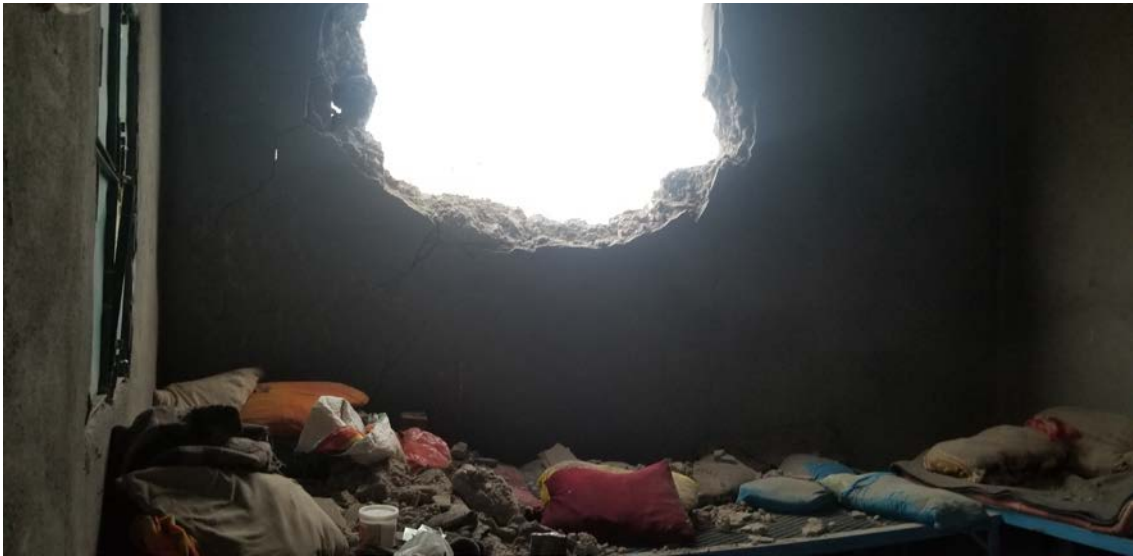
A hole in the wall of the damaged house in Al-Mughal, Hays District, Al-Hudaydah Governorate, photographed on 3 March 2021. © Mwatana.
