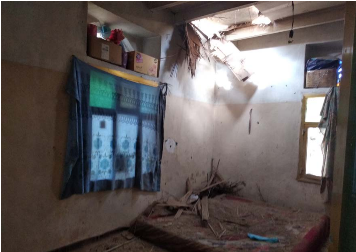
Damaged room in the house in Bir Basha, Old Airport Neighbourhood, Al Muthafar District, Taiz Governorate, photographed on 16 November 2020. © Mwatana.
