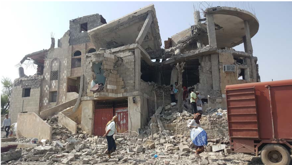
Damaged house in Warazan Area, Khadir District, Taiz Governorate, photographed on 29 June 2019. © Mwatana.
